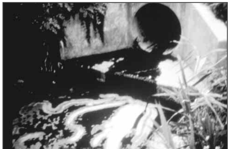
Figure 4.6.4-2. Example of a severe pipe outfall.
