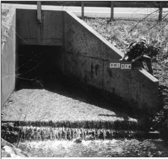
Figure 4.6.5-1. Perched culvert causing fish migration blockage.
