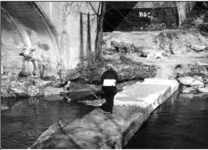
Figure 4.6.3-2. Example of a sever exposed pipe problem.
