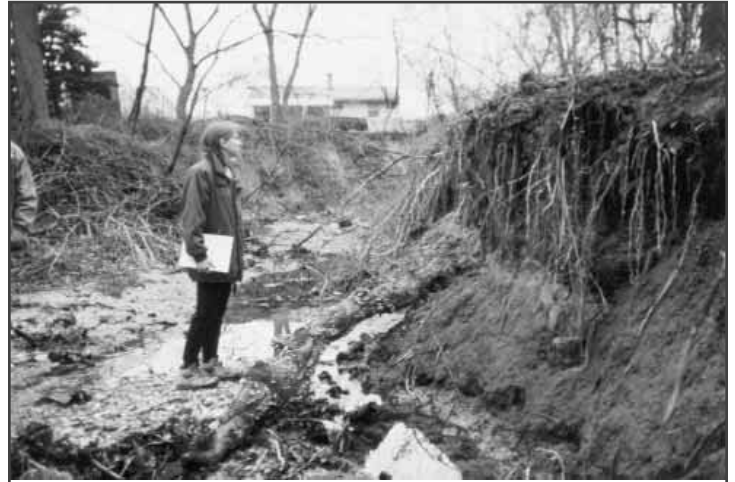
Figure 4.6.2-1. Photograph of a stream erosion site.
